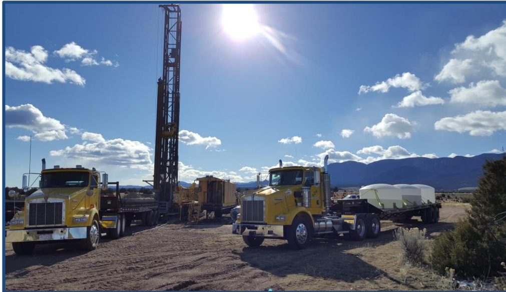
Math Energy Atlas Copco RD 20 Range 3 drill rig on location drilling Austin's C18#2 well
